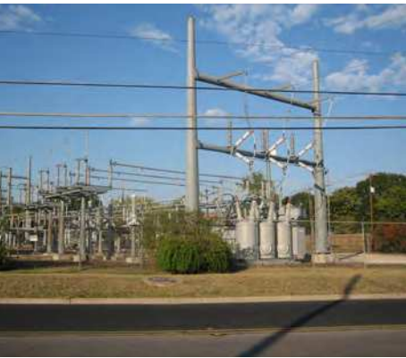
A transformer station in Northeast Austin.
